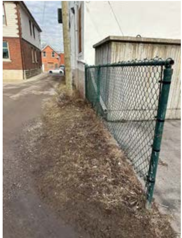
Image 14 Downspout draining to asphalt
