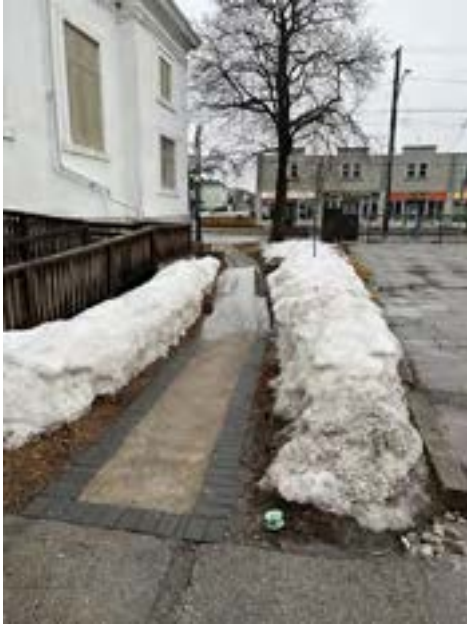
Image 27 Permeable Pathway March 5, 9:05am Water pooling in lowest area
