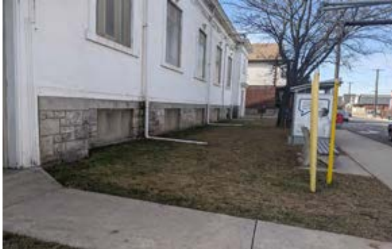
Image 20 Three disconnected downspouts draining to turf
