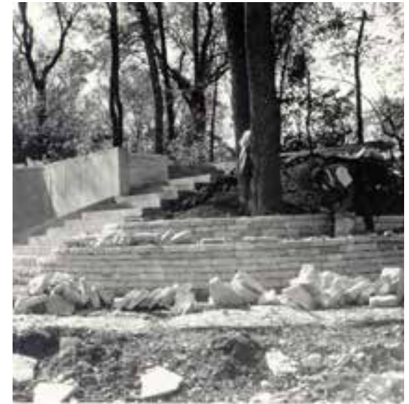
4.2 Landscape construction, Kildonan Park Pavilion, Winnipeg, 1964, CW. Gunter Schoch stayed on site to direct the work crew as they placed stones for the patio, stairways, pond edging and retaining walls.
